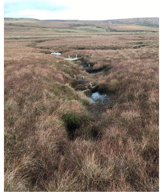
Gully blocking south of A57
